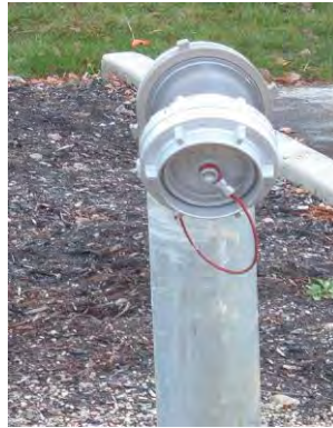
Fire Department Connection
