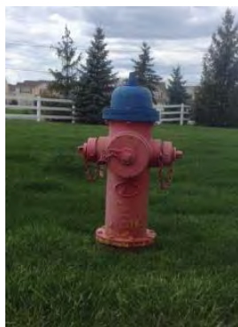
Private Hydrant with OSHA Blue Bonnet
