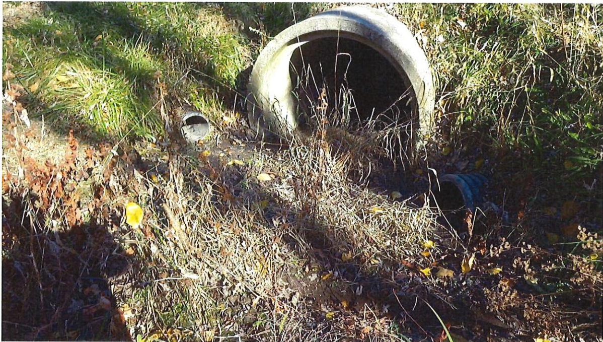
Photograph 8 View of culvert conveying drainage beneath Elliot Road and into Clover Groff Ditch, facing south. (EMH&T 11/10/16)
